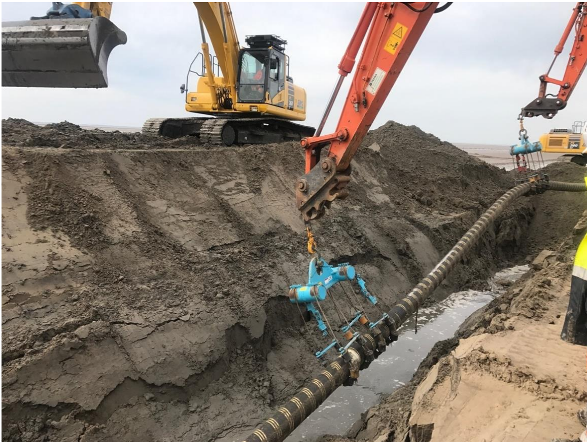
Plate 4.5 Cable being placed in an excavated trench (Walney Extension Offshore Wind Farm)
