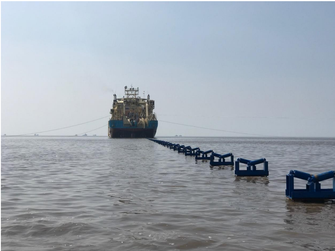
Plate 4.1 Example CLB in position using a mooring system with cable rollers in the foreground (Walney Extension Offshore Wind Farm)
